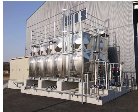
Wastewater treatment facilities
