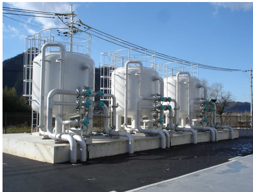
Water supply facilities
