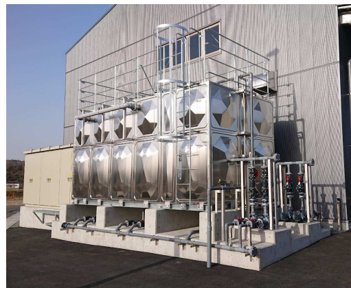
Wastewater treatment facilities
