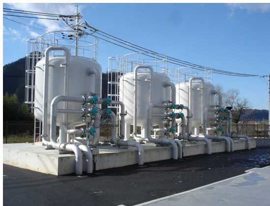
Water supply facilities
